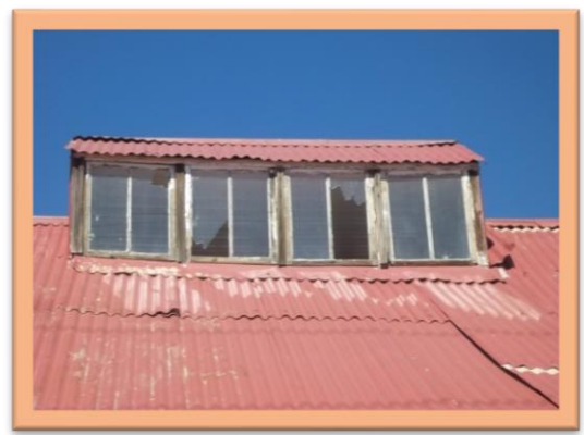
Repairs to roof needed
