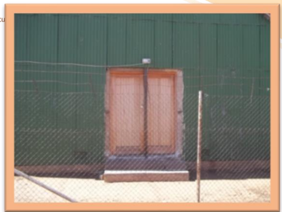
Fence to be upgraded
