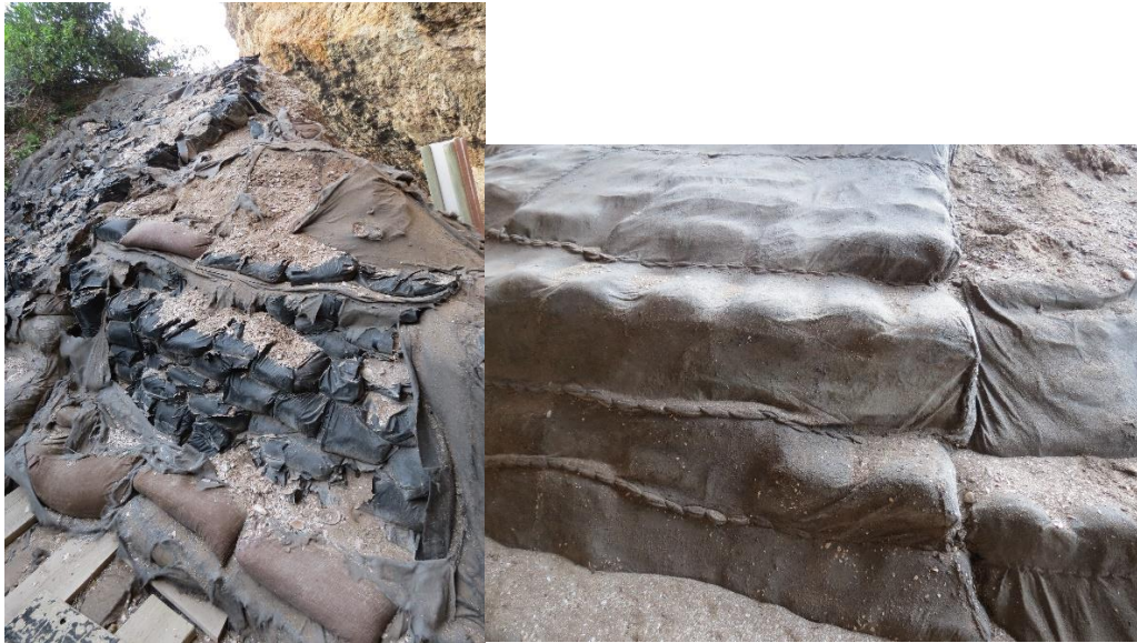
Figure 1. Example of damaged nursery bags and geotextile and example of previous rehabilitation work still in good condition.
