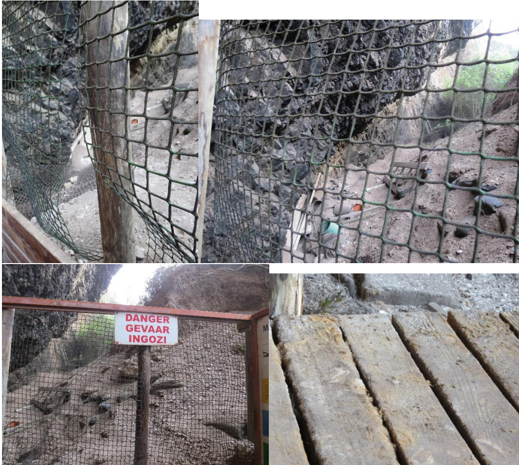
Figure 3. Example of damaged diamond mesh and damaged boardwalk to be sanded.
