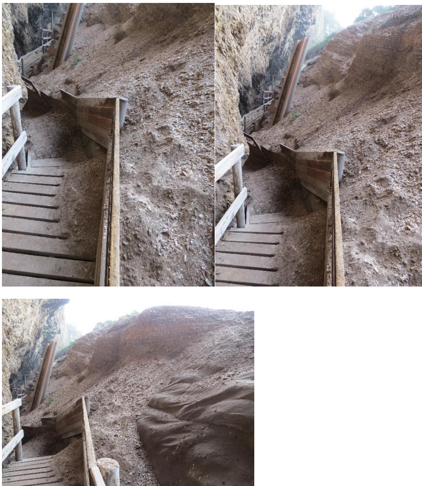
Figure 2. Examples of loose shell deposit to be removed before stabilisation with loffelstein retaining wall.
