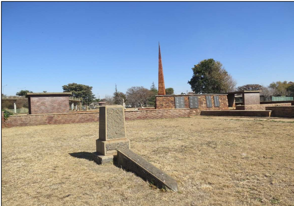
Fig.1 The Obelisk lying on the ground after being falling off the plinth. The appointed service provider must first reinforce the obelisk before mounting it back on the plinth.
