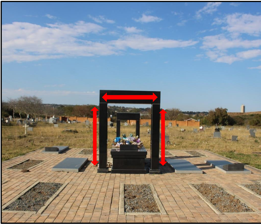
Fig.1 The three pillars that must be removed and replaced with solid polished Zimbabwean granite.
